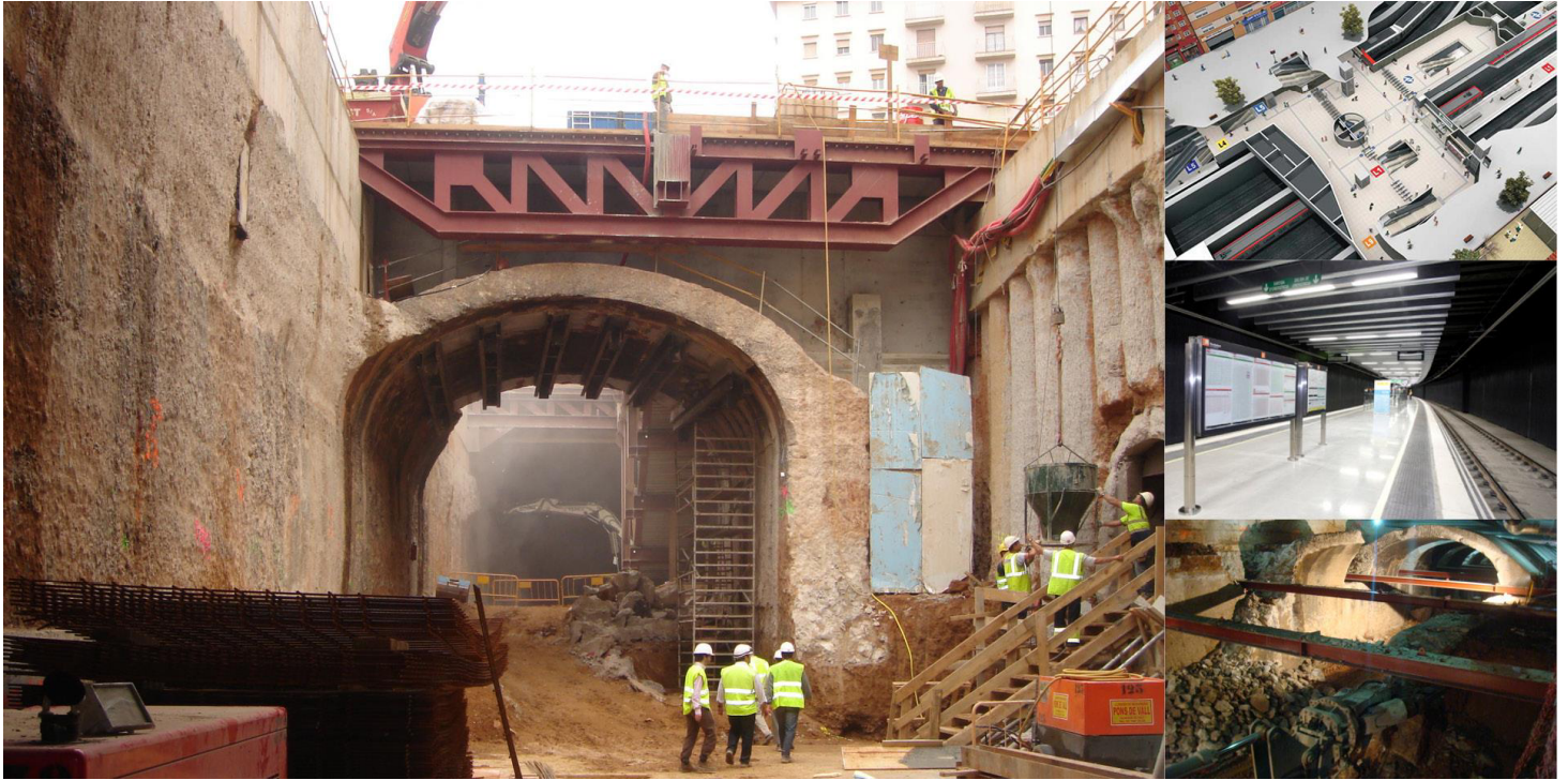
Composite slabs in vestibule, roof built with prefabricated beams and solid slab vaulted roof to be demolished
